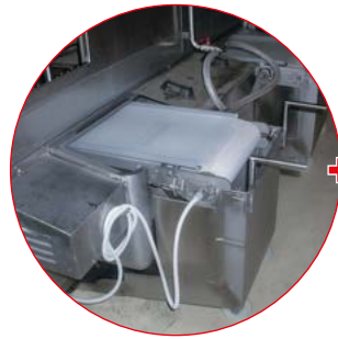
Belt filter to remove particles bigger than 2 mm 2
